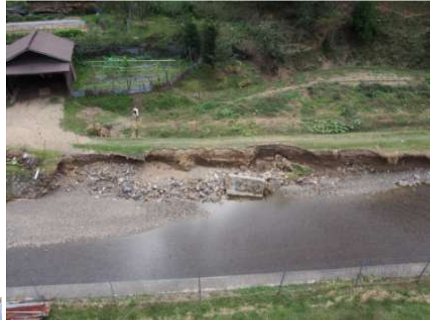
Damaged embankment from UAV
