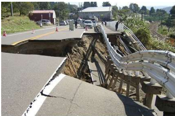
Slope failure due to earthquake After Niigata Pref.
