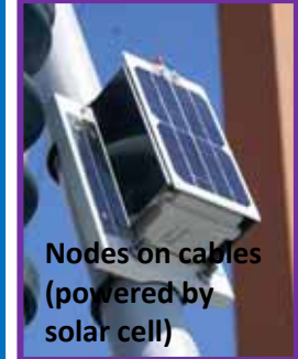
Nodes on cables
