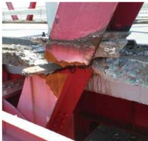
Broken steel, the upper and lower portions are completely divided.
