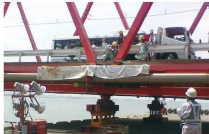
The day after discovery, road administrators were carried out emergency repair work.
